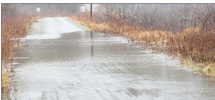
Water covers Blair Road over the cement block culvert during Monday's storm. Submitted photos
