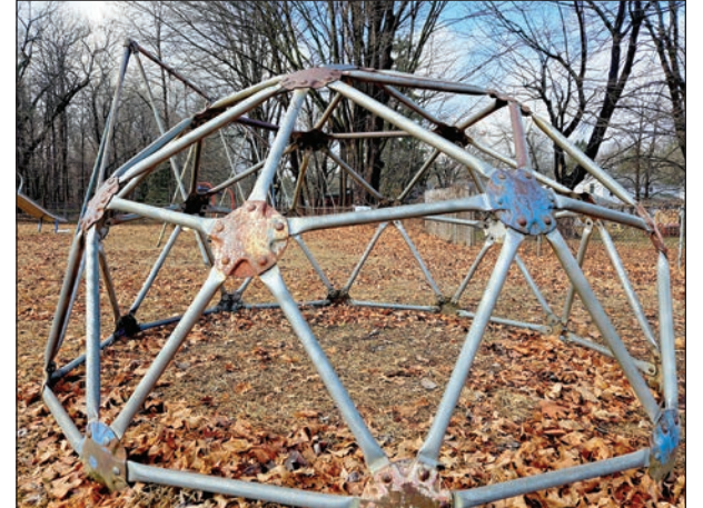
Rusted play structures are evident in the recreation area behind the library. Turley photos by Kathryn Koegel
