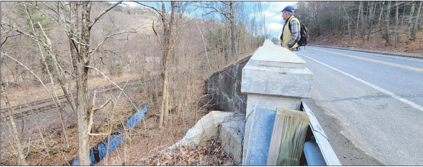
Russ looks down below the bridge. People can see the old railroad as it connects to the Boston and Albany Railroad.
