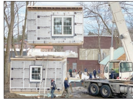
The crane puts a section of the Dwight's ADU on the foundation. Submitted photos
