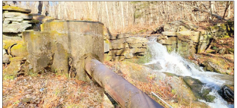
Submitted photos This view of the lower dam shows the penstock to divert water to the mills downstream.
