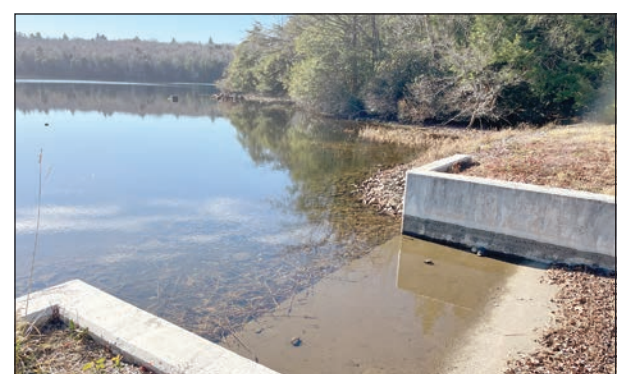
The spillway has not had a flow for several months, according to Water Superintendent Gordon Avery.
