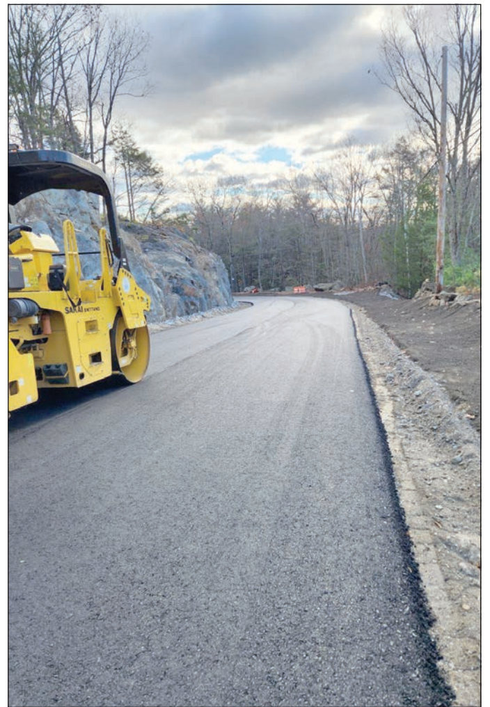
The exposed rock outcrop on left behind equipment is what’s left after curve correction.
