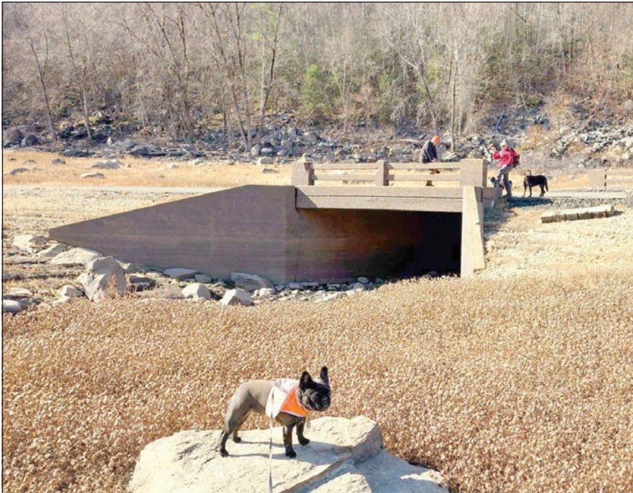
This is a 1953 poured concrete bridge on old Route 8. The Hilltown Hikers and their canine friends explore the area.
