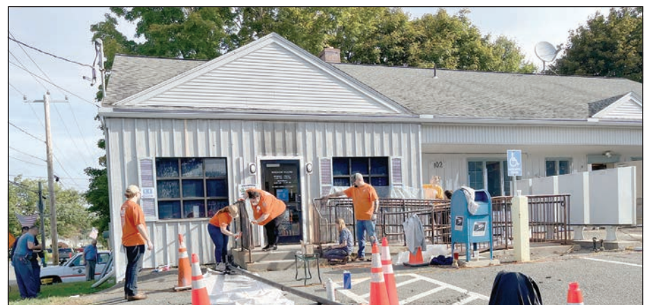
Home Depot employees volunteered and painted the Fire Department Training Center, railings and flagpole.
