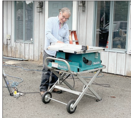
John Piper works on the molding around the doors getting the more complicated work taken care of so work will go smoothly Saturday. Turley photo by Mary Kronholm
