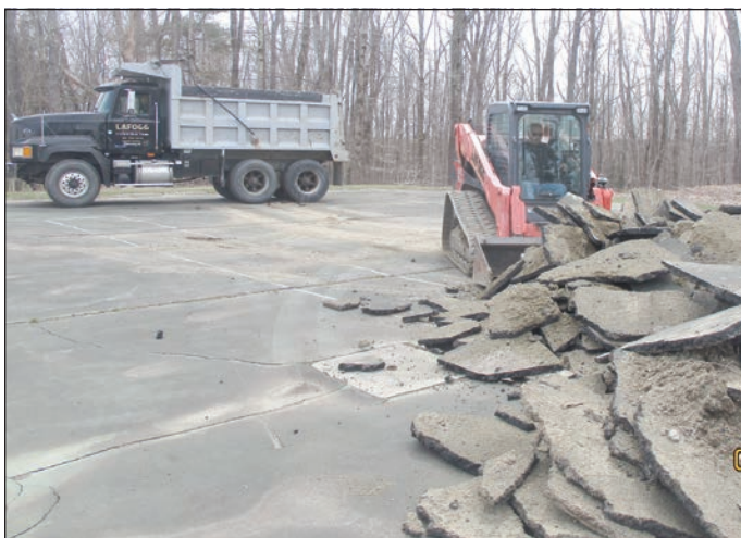
Peter LaFogg of LaFogg & Hathaway Construction in Williamsburg, removes the tennis court asphalt in Goshen center.
