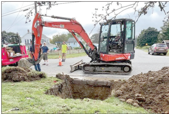
Water Department Steve Grondin, right and Water Department Superintendent Gordon Avery, left, wait for parts to be delivered for a water service repair on Kaolin Road. Photo by Mary Kronholm
