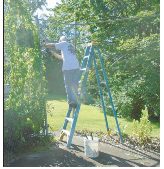
Gary Cunningham removes bolts holding up the chain link fence. Submitted photos
