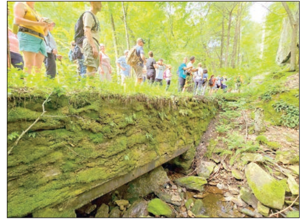
The group stopped at one of the stone bridge culverts along Munn Brook built during the Colonial era.
