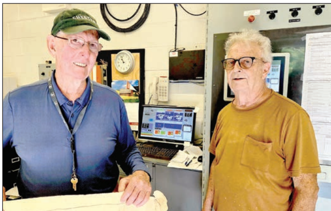
Chester town water commissioner Bob Daley with water plant operator Jim Gobeille in the treatment plant Sunday. Daley holds the 1913 plan for one of the two reservoirs supplying the plant with the modern system in the background.
