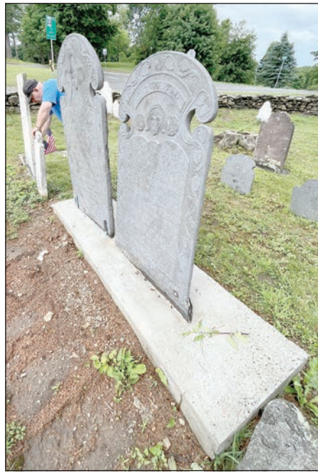
Two headstones in the Old Burial Ground have been properly set in a three-foot deep cement footing.
