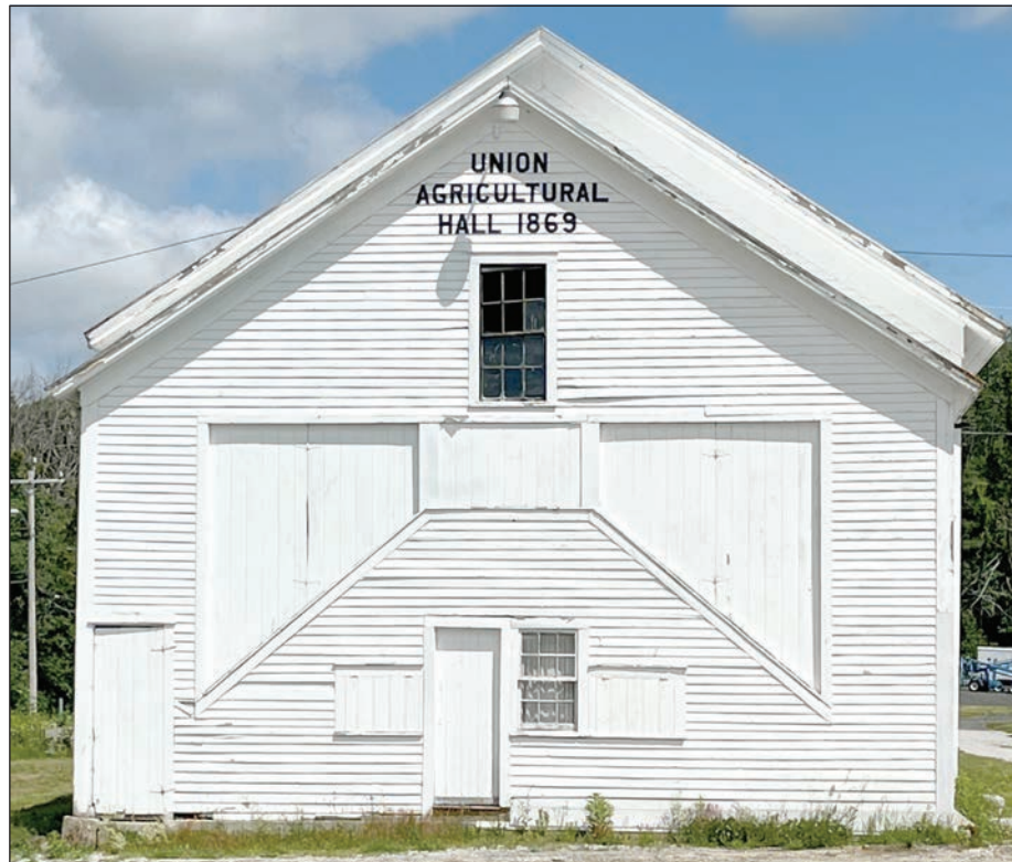
The Agricultural Hall at the Blandford Fairgrounds, a new roof is the Blandford Fair Preservation Association’s first priority. Turley photos by Mary Kronholm
