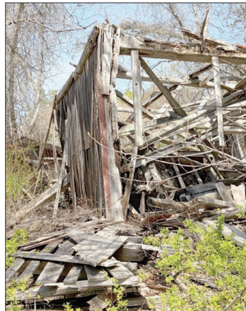
This shows a collapsing barn located on Montgomery Road in Montgomery.
