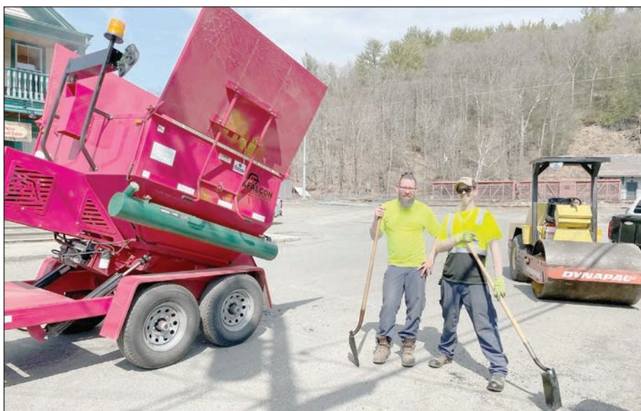
Chester Highway Department workers Chris Brown, from left, and Paul Hathaway (right) use the town’s new Asphalt Recycler and Hot Box Trailer to fill potholes with hot patch along Main Street in Chester Village.
