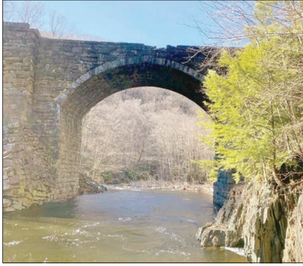
This is the 65 foot Keystone Arch Bridge. Photos by Karen McTaggart, Liz Massa and Paul Normand
