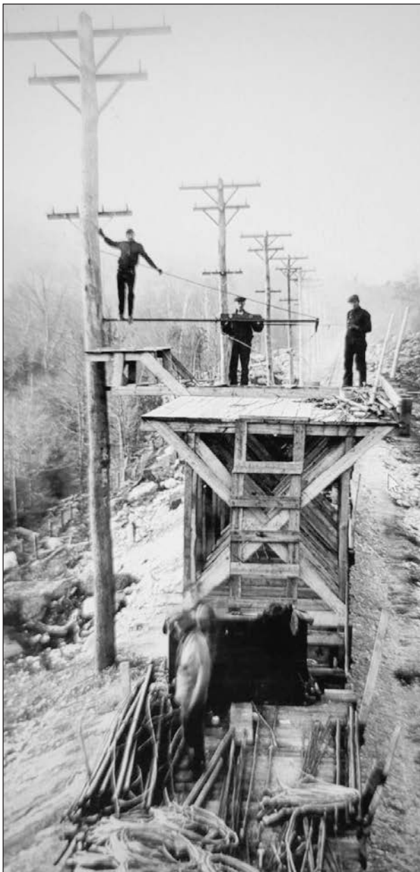
The Tower Car used to attach the cross bars and insulators to the poles.
