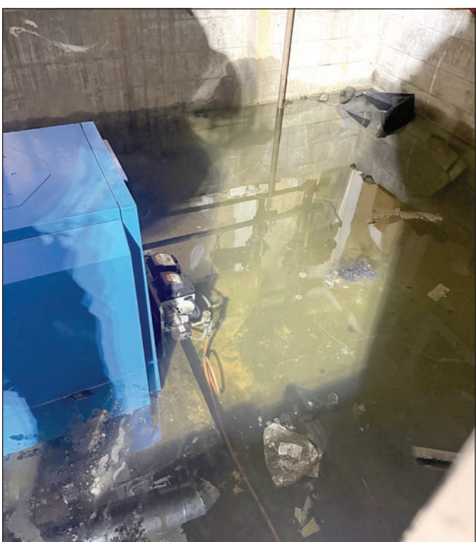
Standing water is shown in the boiler room in the basement of Stanton Hall. The boiler failed sometime during the March 21-22 weekend.
