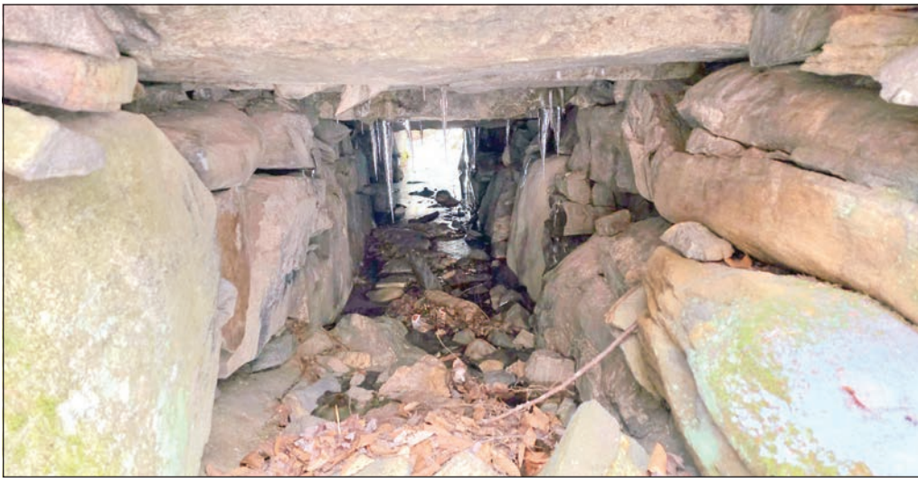
This culvert on the Chester and Becket Railroad was made with Bartlett Quarry granite.
