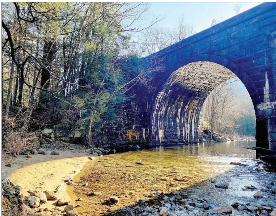
The Keystone Arch Bridges is shown in a snowless January on part of the Wild & Scenic Westfield River.
