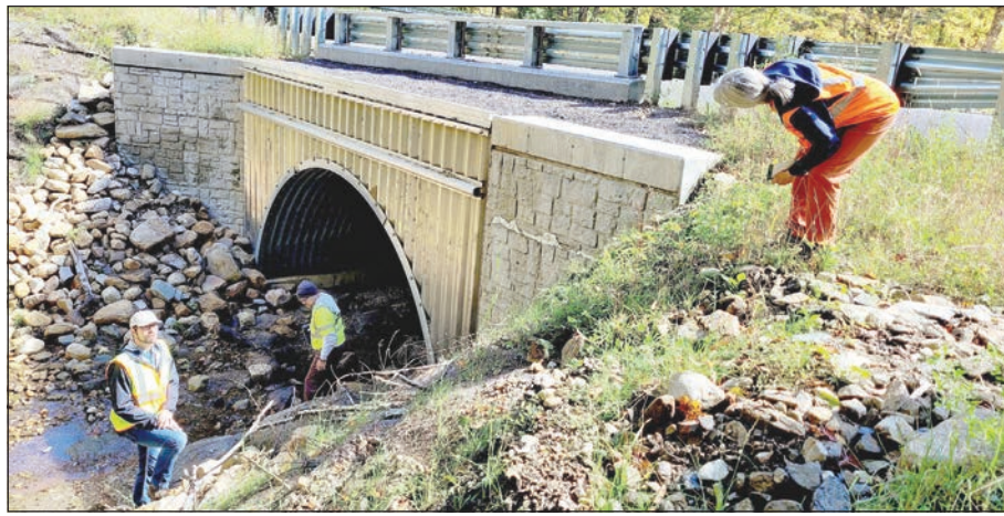
Cindy Delpapa, outgoing chair of the Wild & Scenic Westfield River Committee, inspects a reengineered culvert funded by the committee
