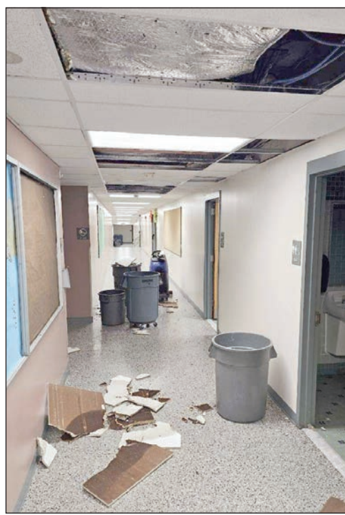
The Gateway Regional Middle High School roof will require extensive repairs in the next few years in order to protect the facilities and safety of students and staff. Barrels collect water leaking from the rood during a rainstorm.
