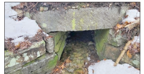
Notched wedge marks from the granite being quarried are visible in a lintel stone placed over the stream culvert for the railroad.
