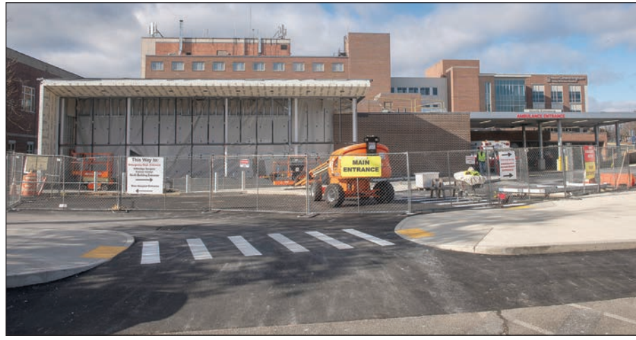
The ongoing construction at Cooley Dickinson Hospital in Northampton to expand the Emergency Department. Submitted photo
