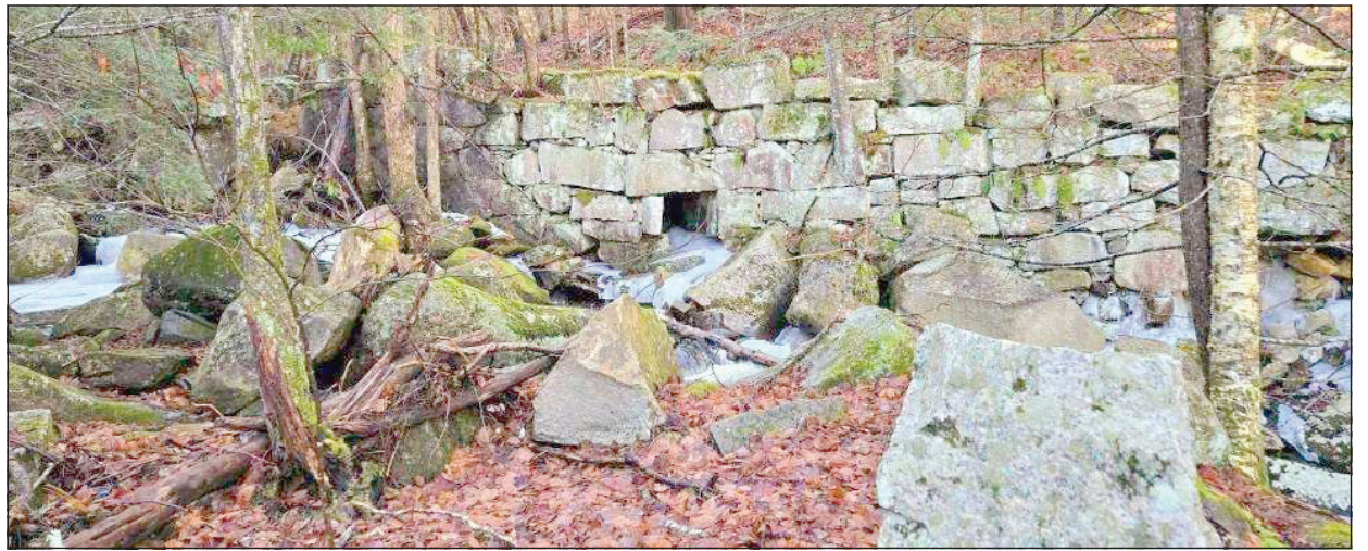
This is a view of the Granite retaining wall for Cushman Brook. The railroad bridge went over the over the brook at this point. Note the stone culvert built into this wall for old Mitchell Road on the other side of the wall.
