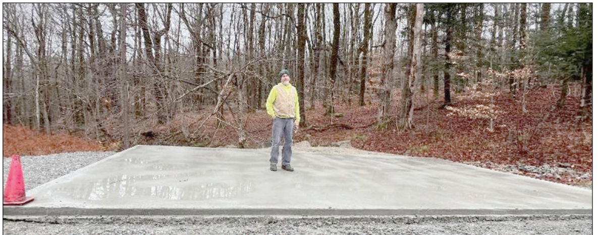
Board of Health Chair and Transfer Station Supervisor Bret Hartley stands on the cement slab foundation of the new Swap Building at the Transfer Station. Turley Photo by Mary Kronholm
