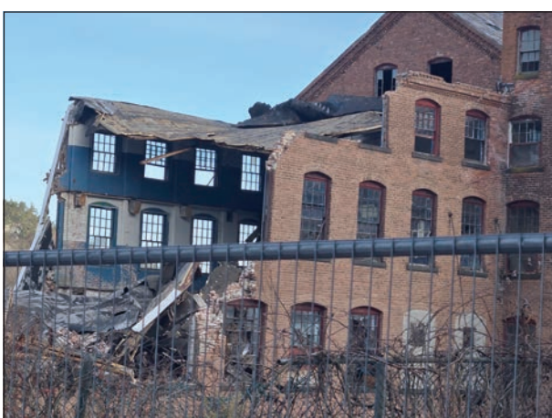
Strathmore Mill #1, located in Russell, collapses on Nov. 11.
